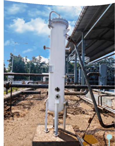
Fuel Gas Scrubber
