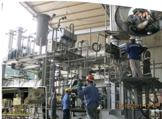
FAT for Burner Management System
