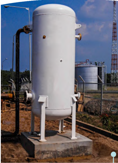
Air Receiver Tank
