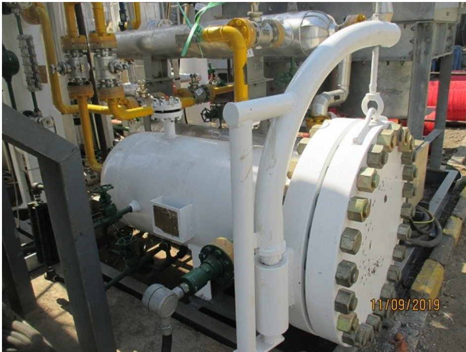
Gas Blower & Housing
