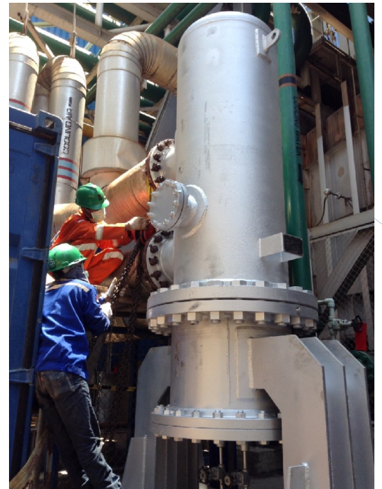
Installation RCA Cooler
