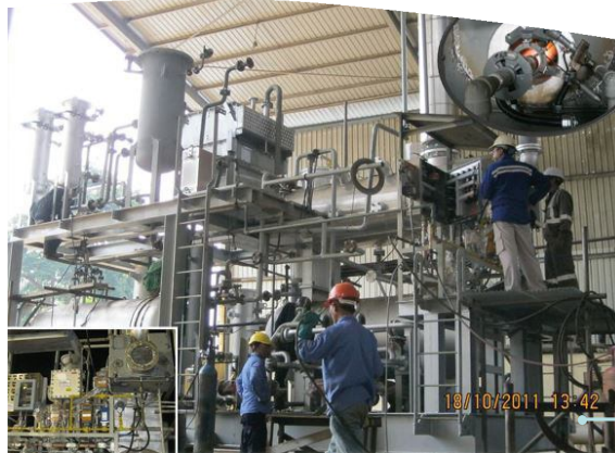
FAT for Burner Management System
