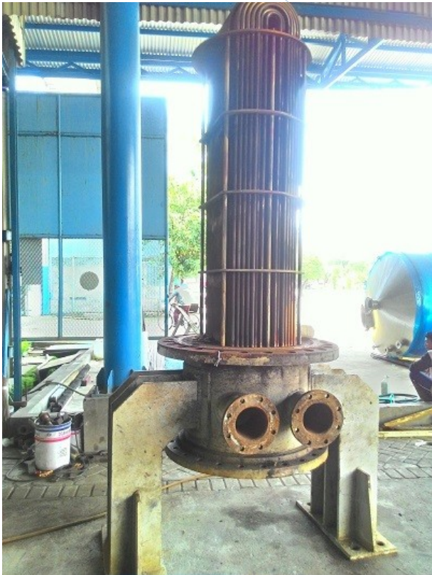
RCA Cooler existing
