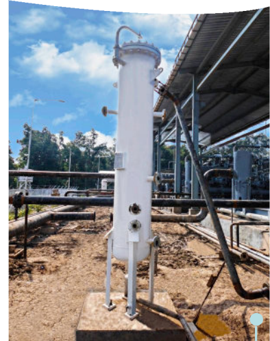
Fuel Gas Scrubber
