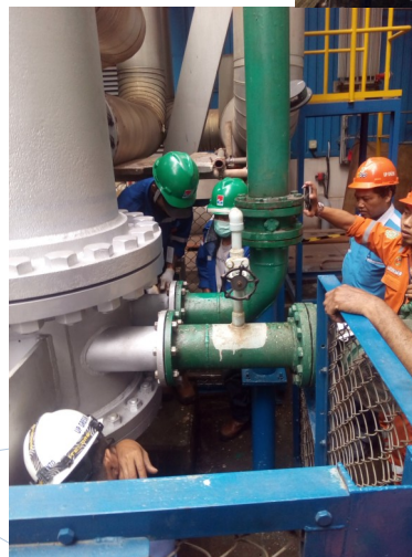
Inspect connecting flange by user
