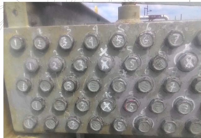
Result Leak Test Header Box
