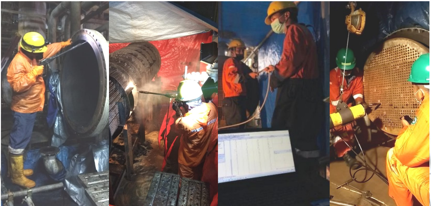
Cleaning Shell Side
